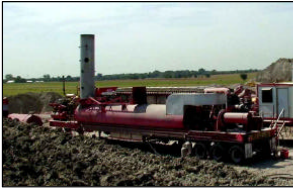
Thermal Treatment Unit
